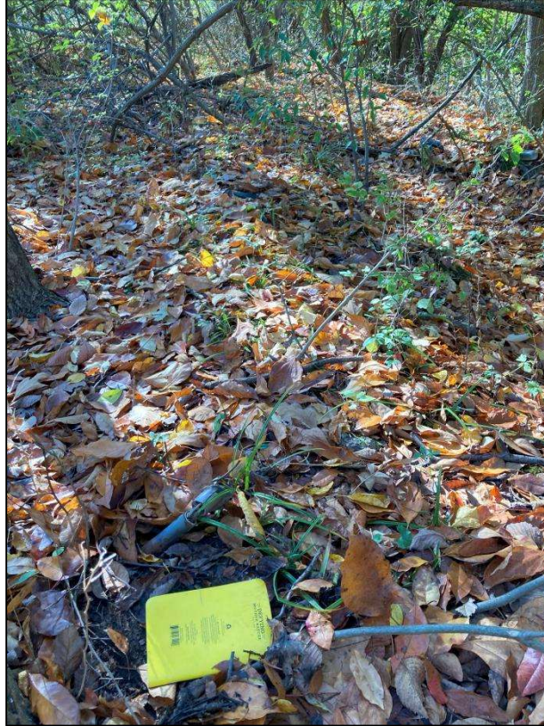
Figure 15. Detail of defunct electrical utility along Townsend Road (facing southwest). Notebook included for scale.
