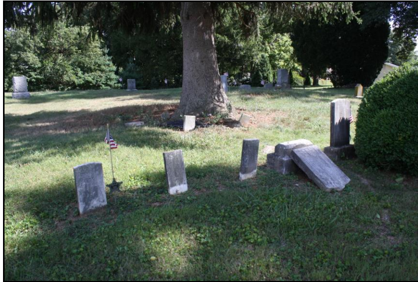
Figure 33: Gravemarkers with atmospheric staining, biological growth, and displacement near Zion Union Cemetery south elevation; Photo view: Southwest; Photographer: Jason Harpe; Date: September 19, 2023.
