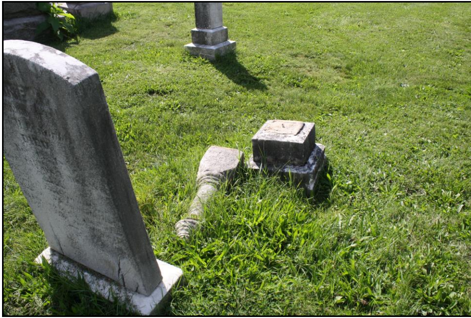
Figure 57: Displaced upper section of a pedestal tomb; Photo view: West; Photographer: Jason Harpe; Date: September 20, 2023.
