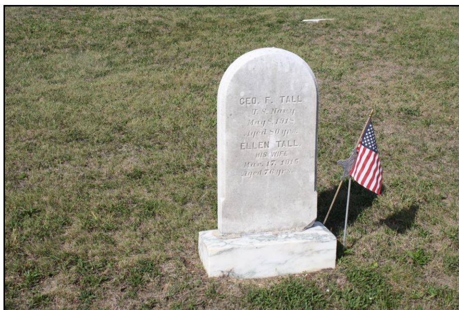
Figure 42: Marble die-on-base gravemarker for George Tall (d. 1918) and his wife, Ellen Tall (d. 1915) showing original cementitious materials used to join the die to the base, as well as some modern inappropriate repair materials; Photo view: West; Photographer: Jason Harpe; Date: September 19, 2023.
