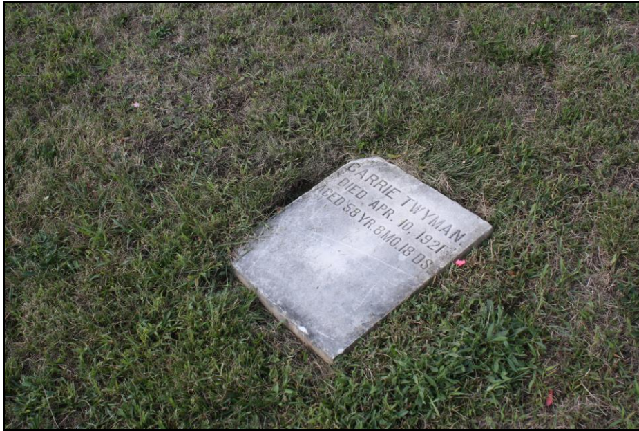
Figure 40: Displaced marble tablet for Carry Twyman (d. 1921); Photo view: West; Photographer: Jason Harpe; Date: September 19, 2023.
